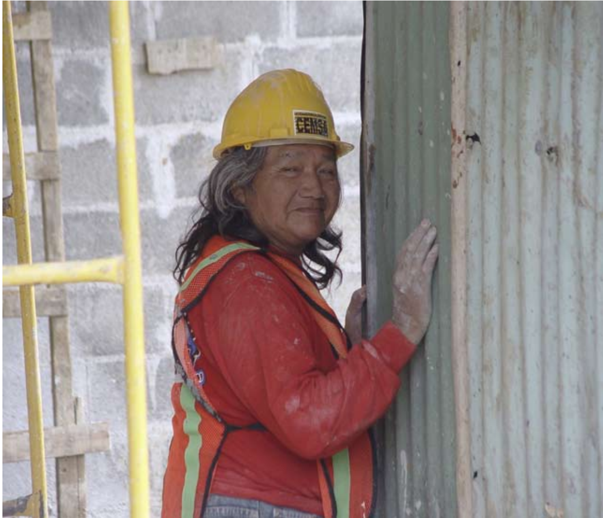
A Nicaraguan worker on the building site for a property development in Heredia. "We have no reliable data on the proportion of women in the migrant workforce, but we are seeing a perceptible increase", remarks Joaquin Melendez Gonzalez (CTRN).
